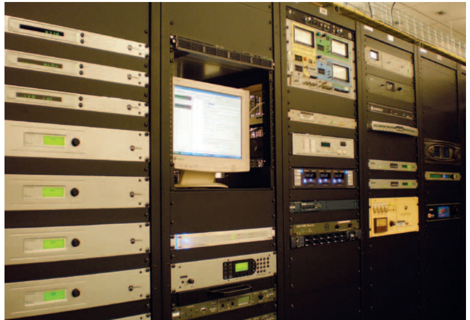
KUNV's rack space in the TOC includes Omnia 6EXi and Omnia One processors, Axia engines and audio nodes, Comrex Access, Arbitron PPM encoders, Public Radio Satellite System hardware, streaming server/encoders and iMediatouch skimmer. Also at work is gear from Sage, Broadcast Tools, DaySequerra, QEI, Orban, Moseley and Belar, among others.
